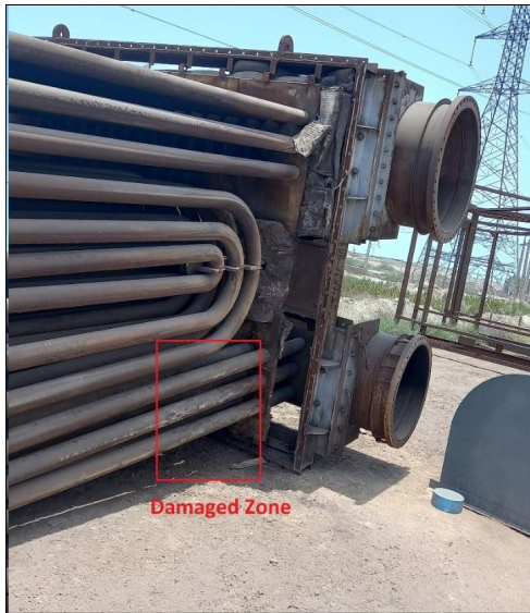
Fig. 8. Damaged sample of the first-stage feed-gas tube bundle.
