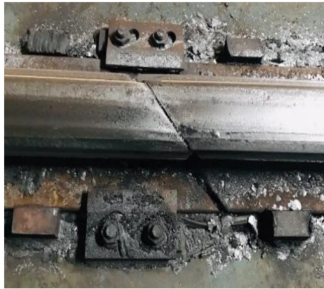
Fig. 11. A sample of the rail gap attachment which is designed and installed in the crane rail of the SKS Company.
