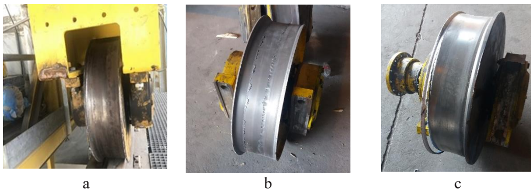
Fig. 3. The wear on the wheel of crane.
