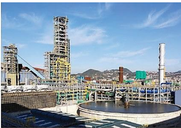
Fig. 5. View of the sponge iron production unit of Algerian-Qatar Steel Company.
